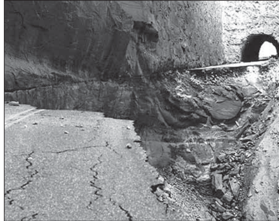
August 8, 1968—Rim Rock Drive washout
