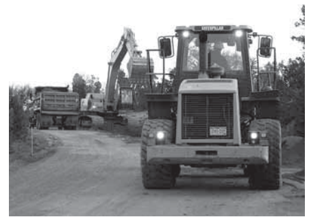
A great deal of heavy equipment was needed in the reconstruction effort.
